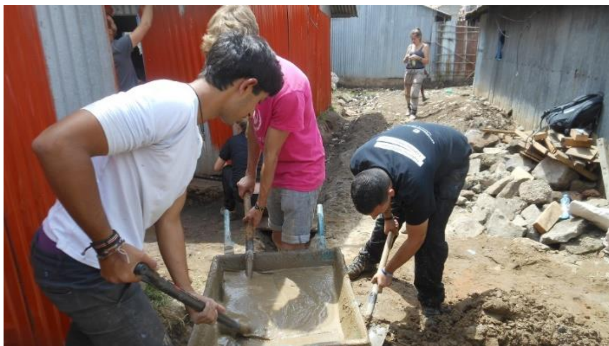
Figure 23 Volunteers mixing concrete for the floor of the kitchen they are building
