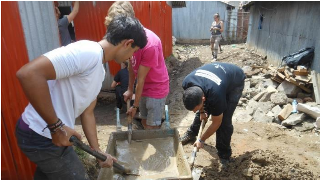
Figure 11 Volunteers Vish, Ramy, and Ned mix concrete for the kitchen floor at Lizpal School
